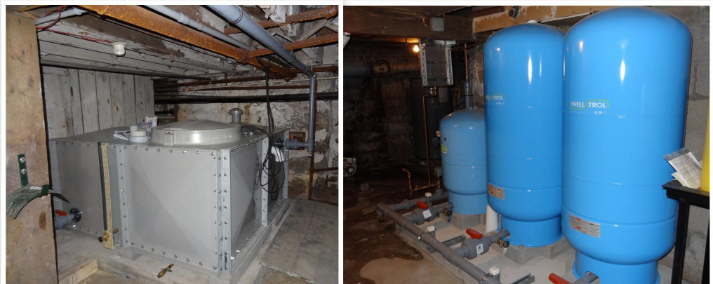
Storage and pressure tanks installed in the basement of the Antlers Main Lodge.
